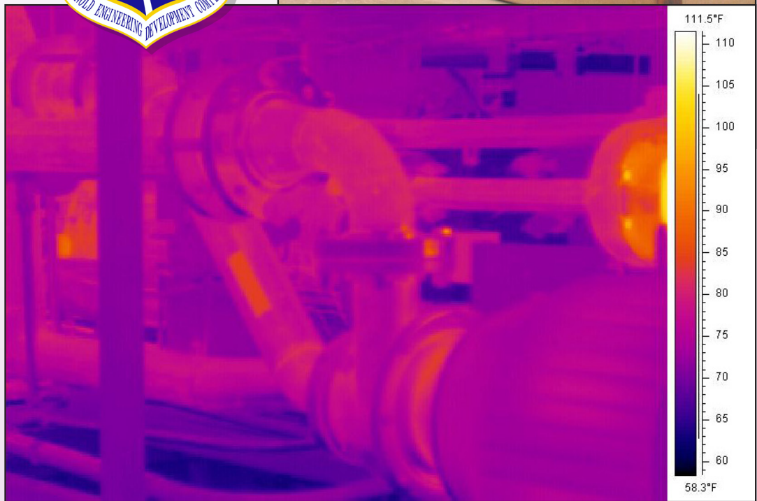
Top: This vintage mid-1980s Air Force liquid flow calibration system was installed at UTSI and utilized to evaluate for needed upgrades.
