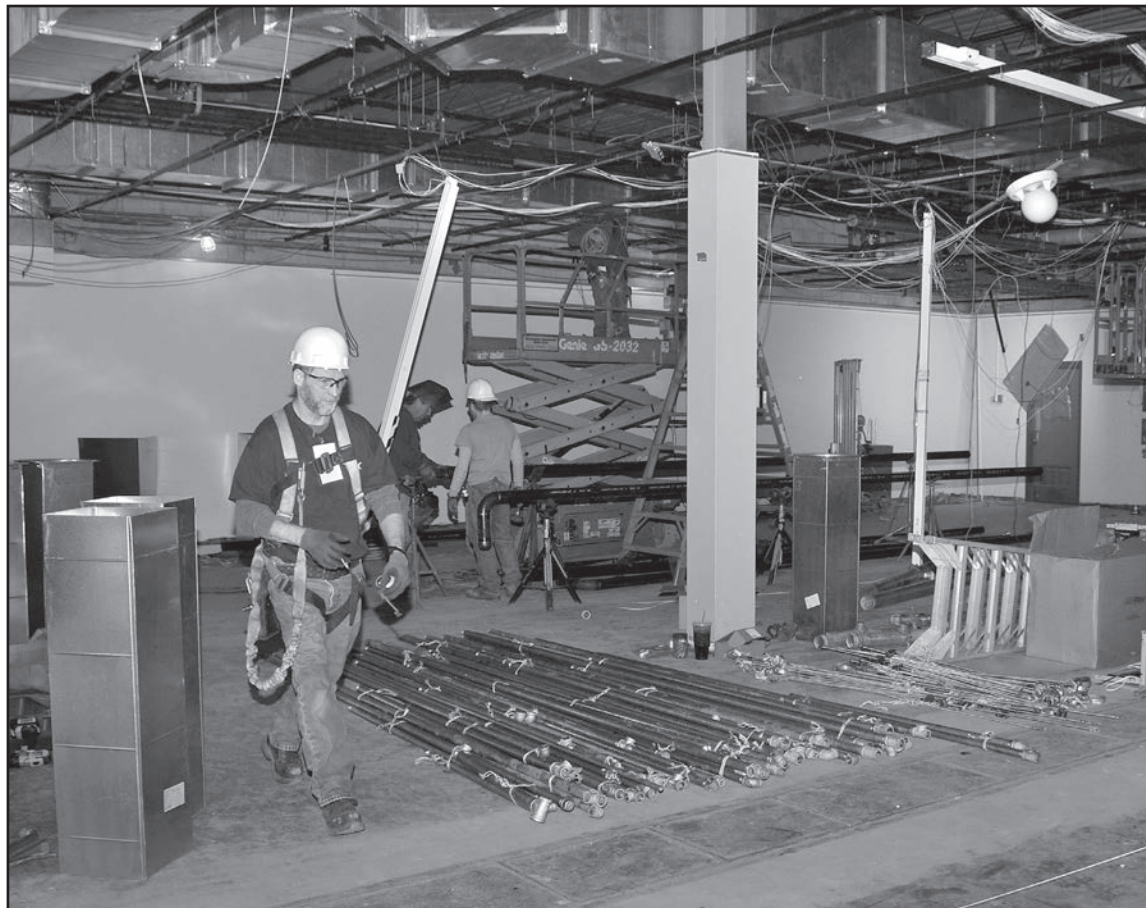
From left, Robert Flanders, with subcontractor Tri-State Sprinkler Corp., works to install a sprinkler system while David Benson and son David with subcontractor Billy Thomas Plumbing and Electric Service, install chilled water piping for HVAC units during the renovation of the Precision Measurement Equipment Laboratory at AEDC. (Photo by Jacqueline Cowan)
