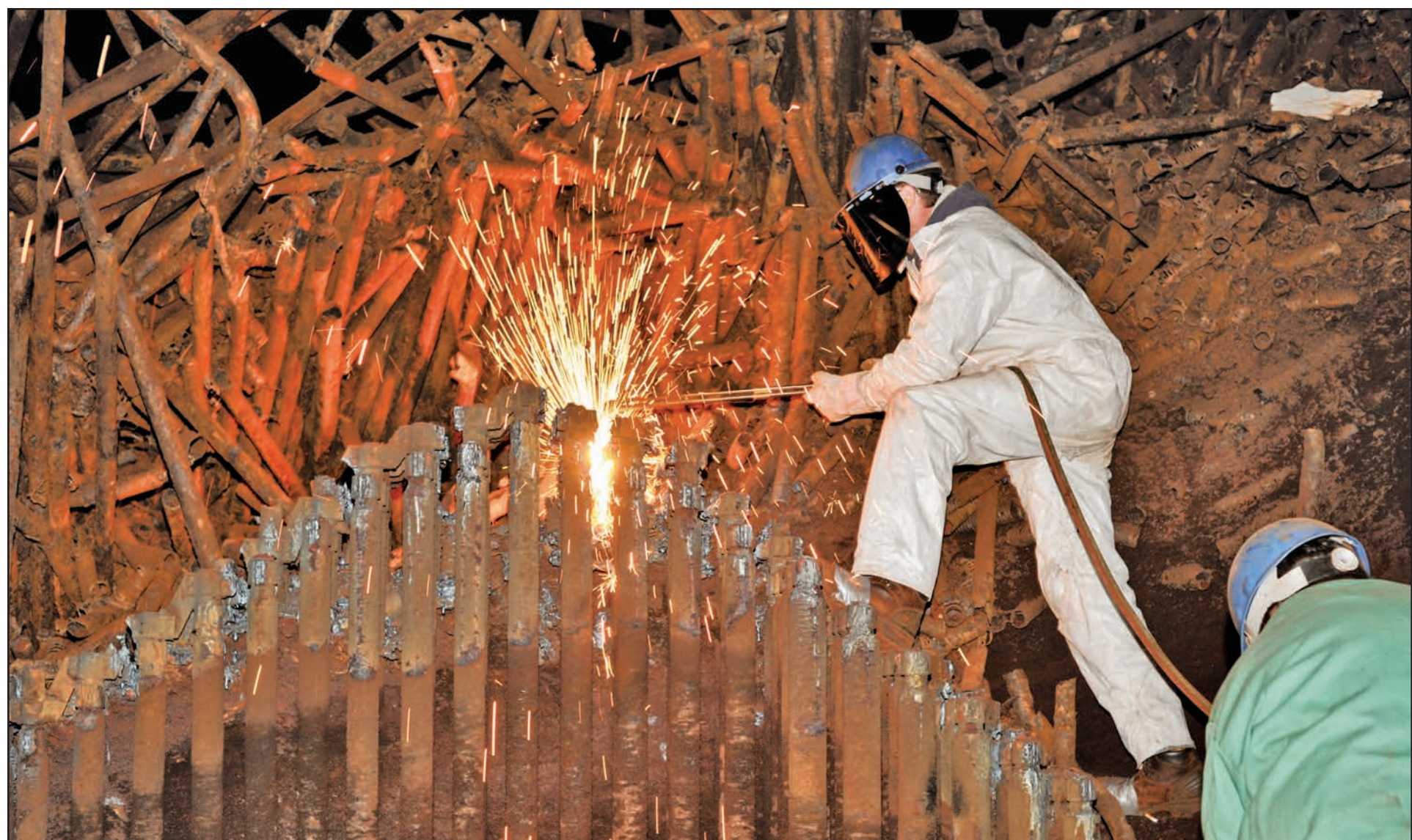
A worker with the National Boiler Service, Trenton, Ga., cuts pipes in the AEDC Aeropropulsion Systems Test Facility (ASTF) EC1 cooler for removal. Once the pieces are removed, new parts will be installed. The cooler assists in conditioning high temperature exhaust generated from jet engine tests. (Photo by Rick Goodfriend)
